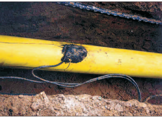
Fig. 5: Stress cracks as a secondary damage in inadequately field coated connections for cathodic corrosion protection
