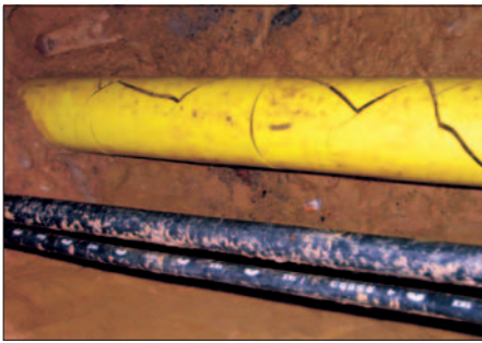
Fig. 3: Polyethylene coating damaged by embrittlement
