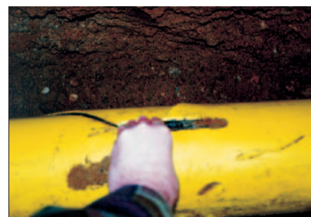
Fig. 2: Cracking due to mechanical stresses
